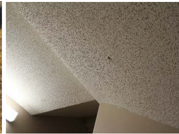
Bullet exited out 2 nd floor ceiling
